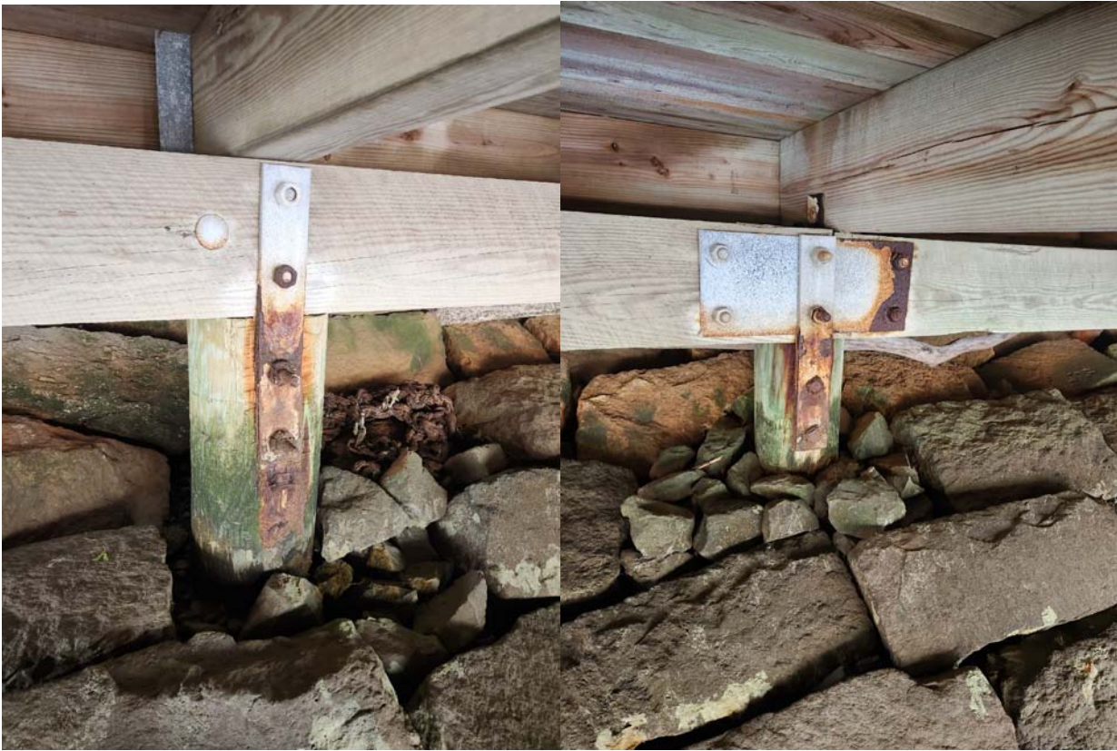
Pile to support beam hardware in (5) locations should be replaced due to corrosion.
